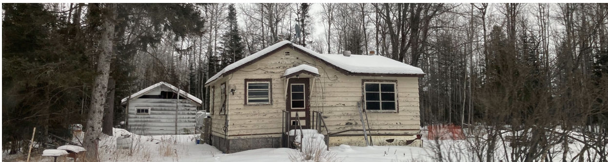
Figure 5.3: Thunder Bay house in need of major repairs
