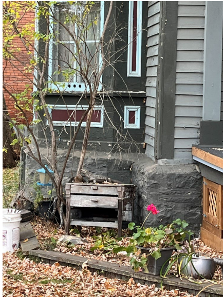
Photograph 15: View of the stone foundation which extends 5 ½ to 7 inches beyond the frame structure of the house and the wood moulding under the bay window on the west elevation (Source: Egis, October 15, 2025).
