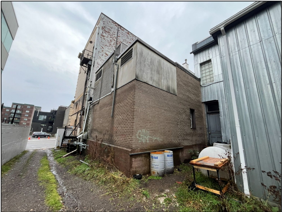
Photograph 5: East and north elevations of the rear of the building (Source: Egis, October 17, 2025).
