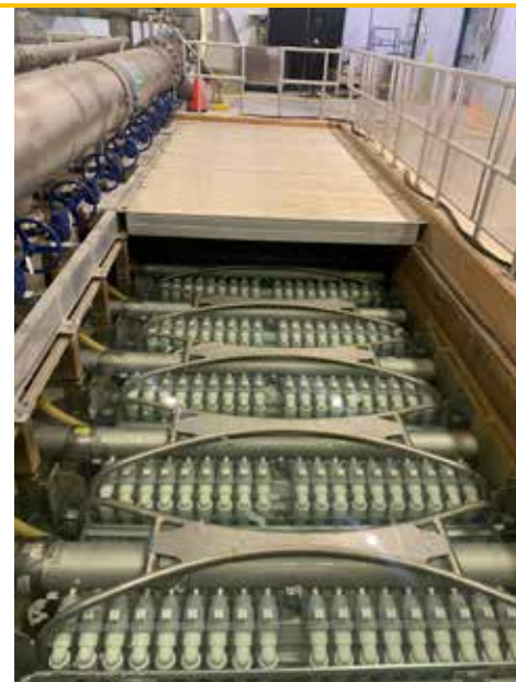
Bare Point Water Treatment Plant filtration system.
