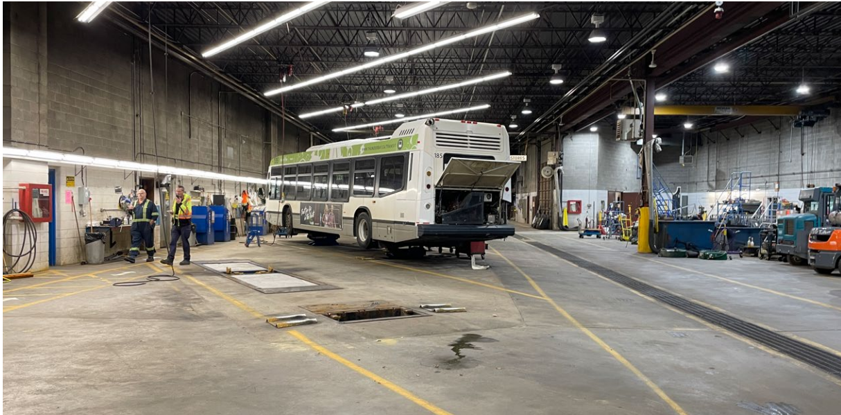
Figure 69. In-Ground Vehicle Hoists at Fort William Road Transit Garage
