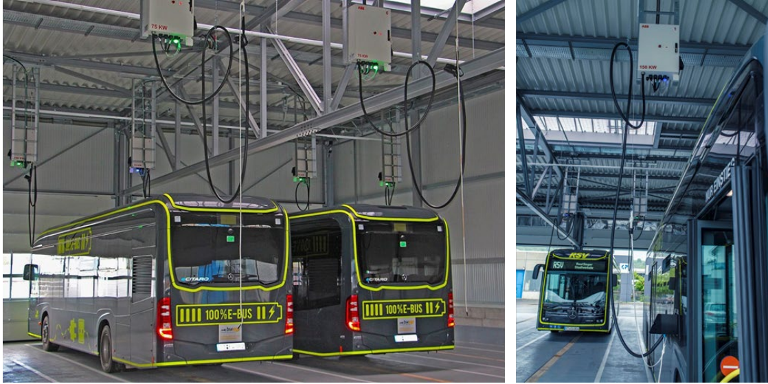
Figure 59. Examples of ceiling mounted chargers
