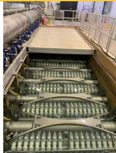
Bare Point Water Treatment Plant filtration system.
