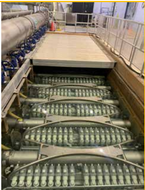
Bare Point Water Treatment Plant filtration system.
